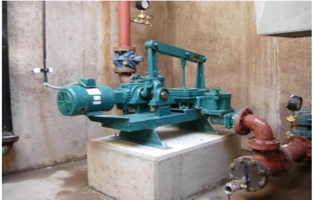
Installation of Mud Sucker 4BW-EC Series Diaphragm Pumps.
