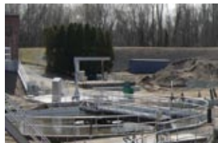
The Glastonbury Water Pollution Control Facility has undergone an extensive upgrade and expansion in recent years.
