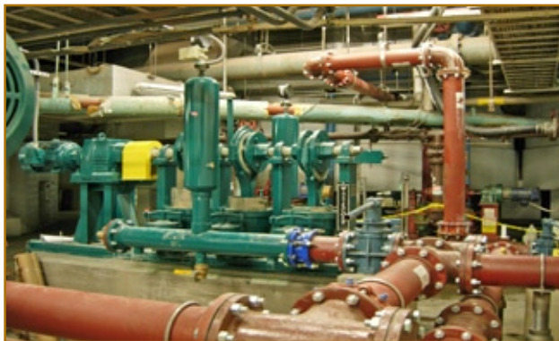
Ossining replaced two existing plunger pumps with the next generation Wastecorp Plunger Pump HPE-1143 Series.
