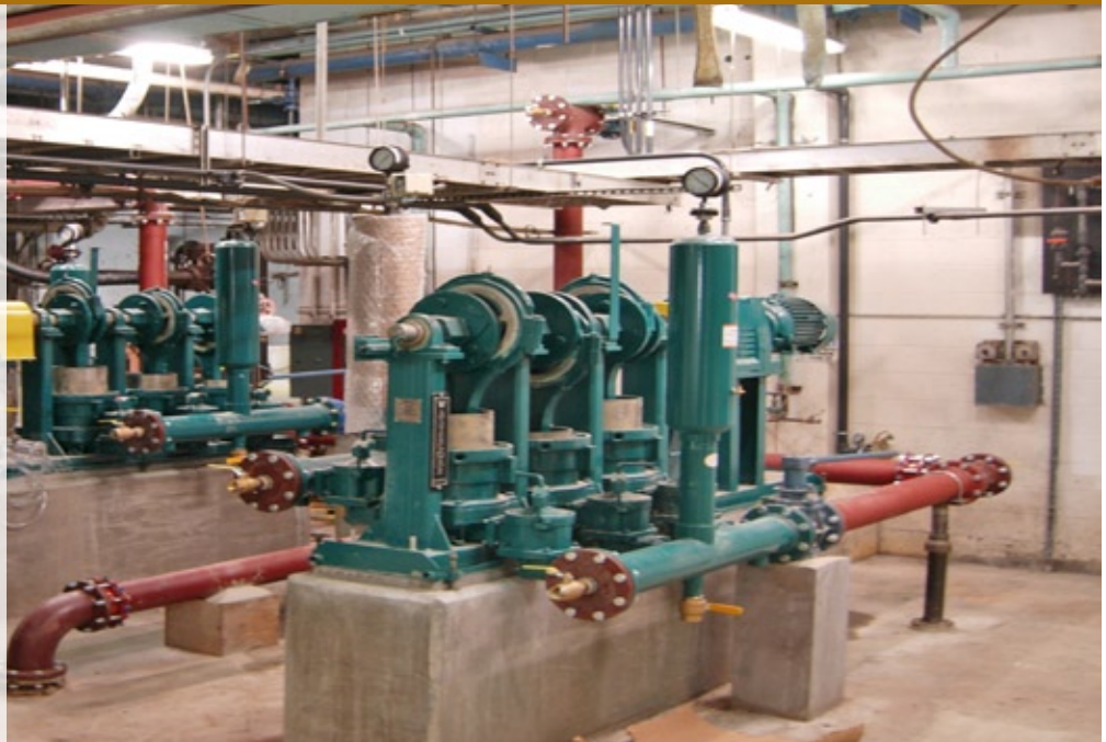
Pump installation day, Wastecorp HPE-1143 Plunger Pumps in New York
