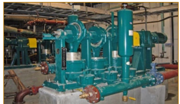
With protective coatings, guided plunger assemblies and gauges, Ossining will enjoy decades of heavy duty sludge transfer services.
