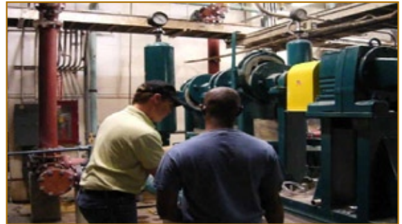
Wastecorp working with the mechanical contractor on installation day, Ossining Dept. of Public Works.
