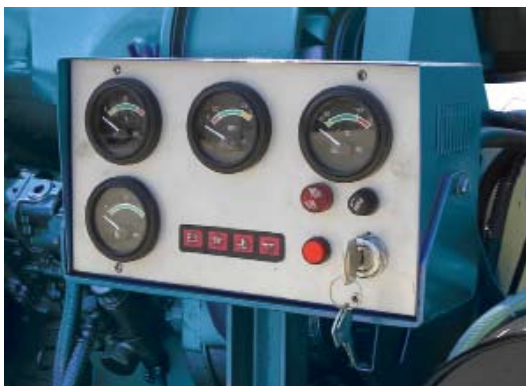
Shown: Deutz diesel engine panel with automatic start and lockable controls during unsupervised operation.
